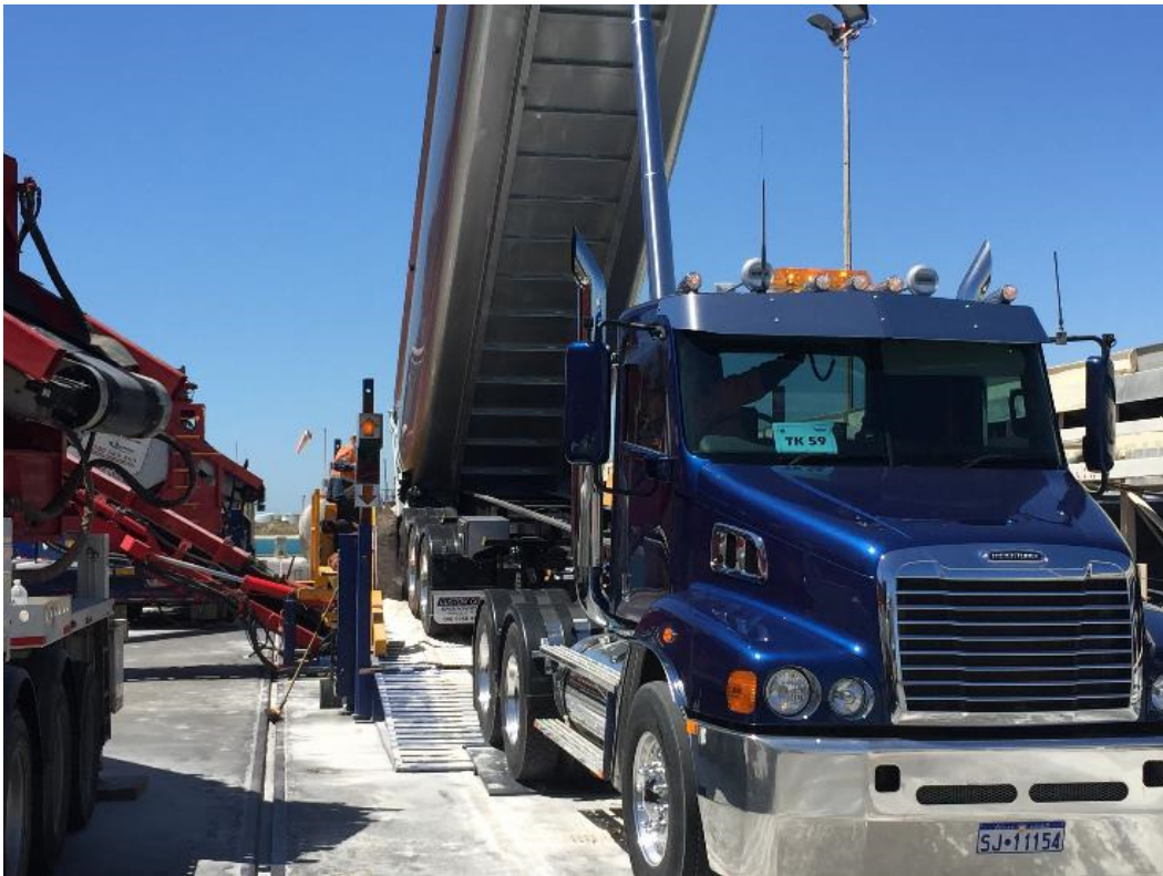
Truck Hopper with light communication system installed to avoid trucks overfilling hopper
