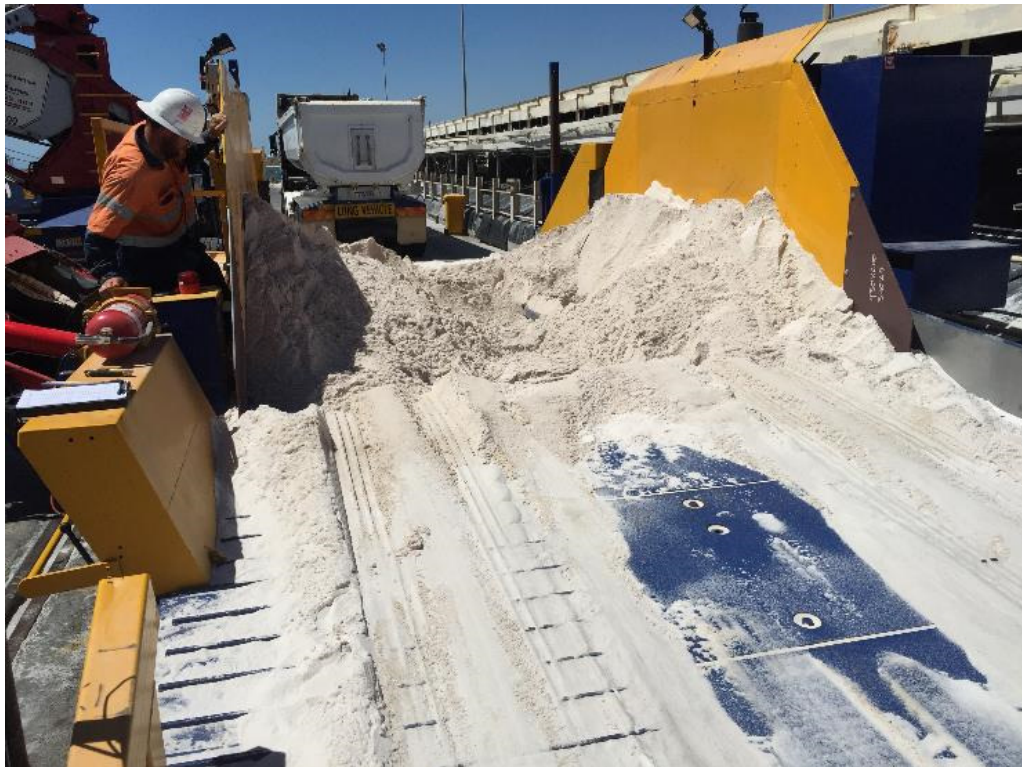
Truck Hopper installed with extended side guarding to reduce spillage and improve containment
