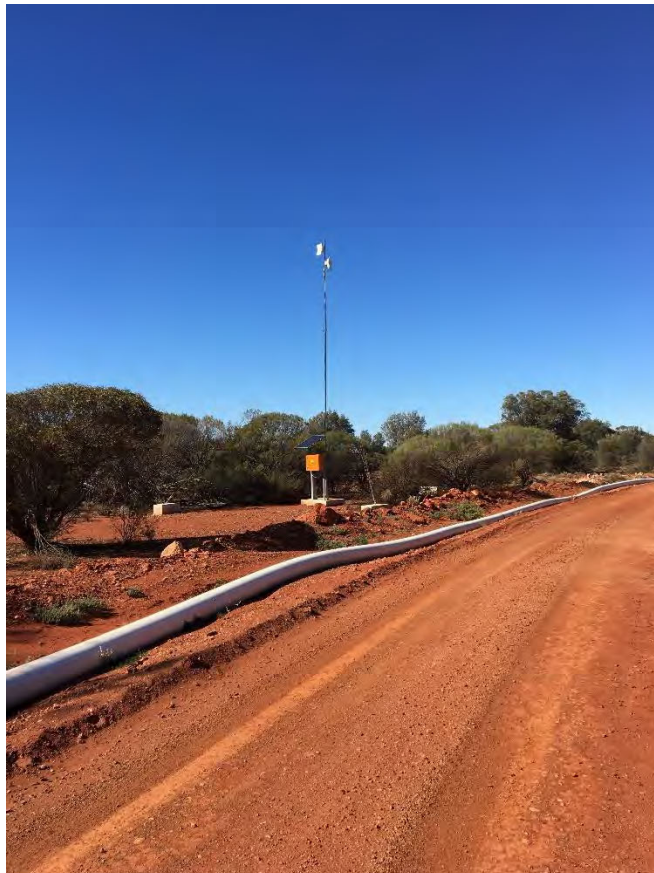
Figure 1: Telemetry receiver tower linked to leak detection system
