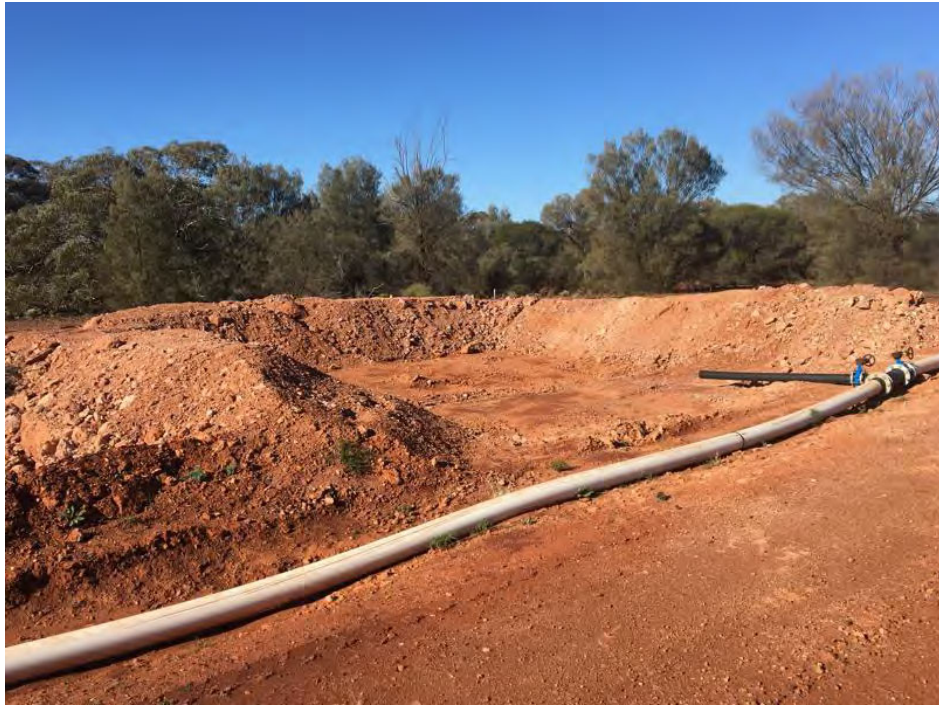
Figure 3: Example of a catch sump located on the Riverina to Lady Gladys dewatering line
