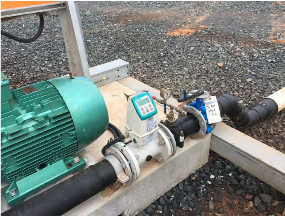
Figure 6: Staging Tank Meter
