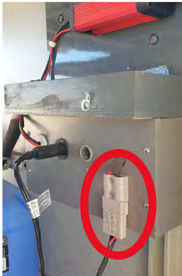
Photograph 5: Electrical connection for pump.
