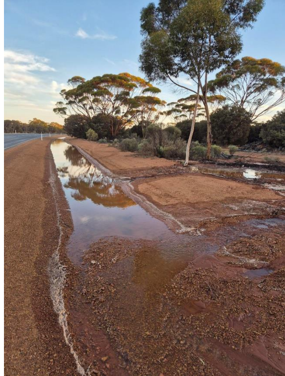
Photo-02 – Water from the trench overflow toward the V drain on the side of the road
