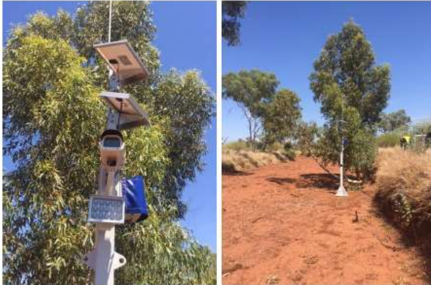
Figure 2: Wetting Front Early Warning Point gauging station (already in place)
