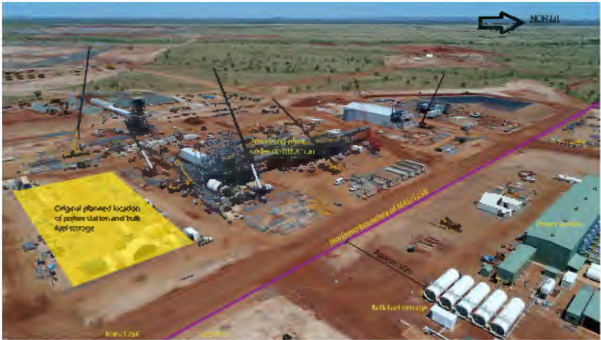
Photograph 1 – Construction location of the Power Station and Bulk Fuel Storage area on L45/417
