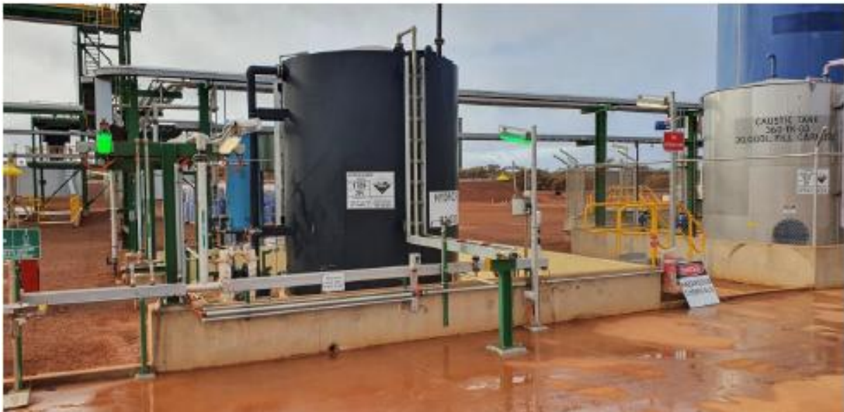
Figure 15: Indicative reagent or chemical storage (hydrochloric acid tank bunding)
