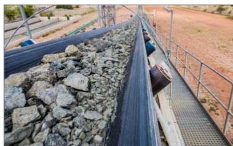
Monitoring conveyor belt - deployment of Xi 80 as an efficient tool for fire safety
