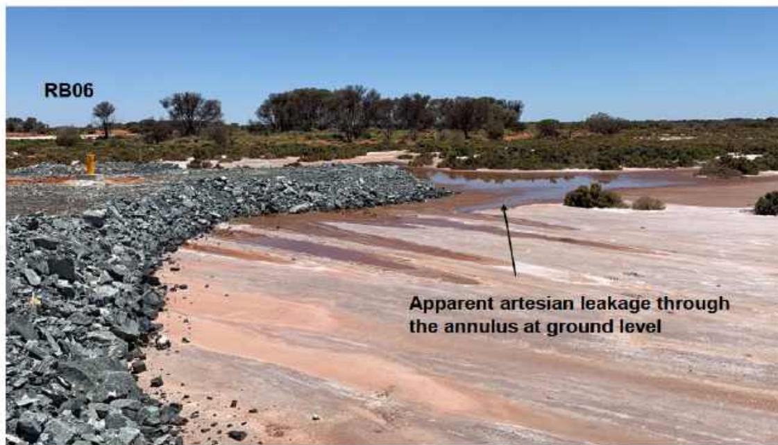
Figure 4-2 Picture of leakage at the base of the causeway at RB06.
