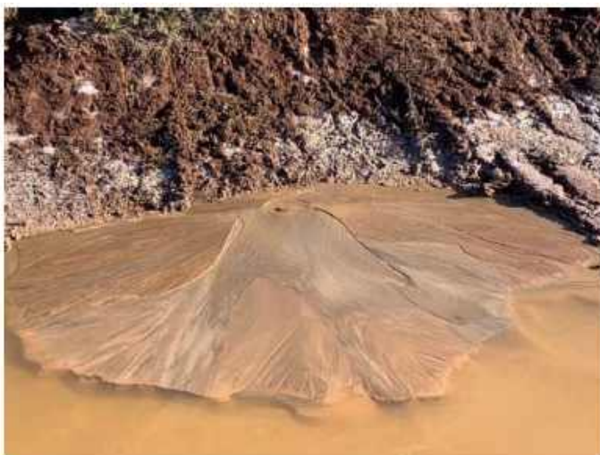
Figure 2-3 Sand boil in the toe drain near RB03 on 27 Jan 2021 (Golders 2021)
