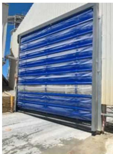
Figure 4: Automatic roller door
