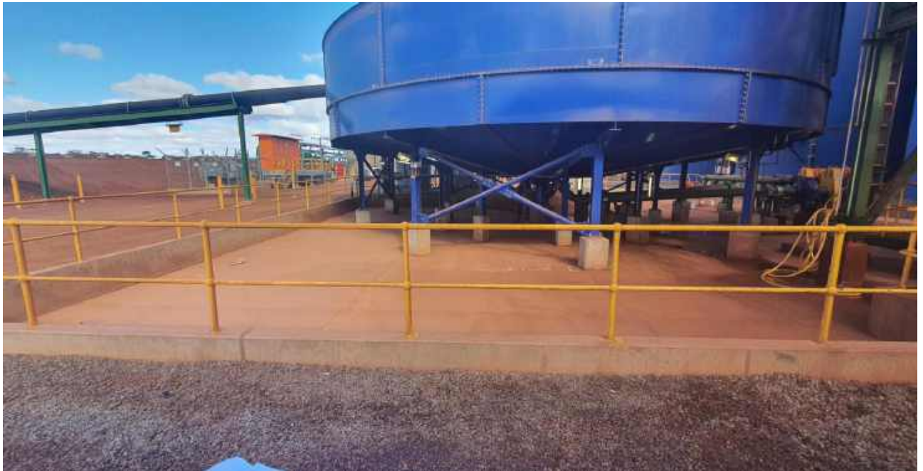
Photo 7 CIP circuit bund – tailings thickener
