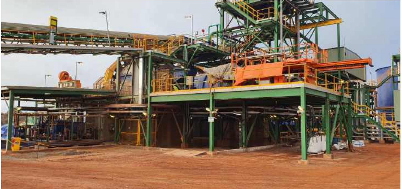
Photo 1 SAG and Ball Mills on bunded concrete pad
