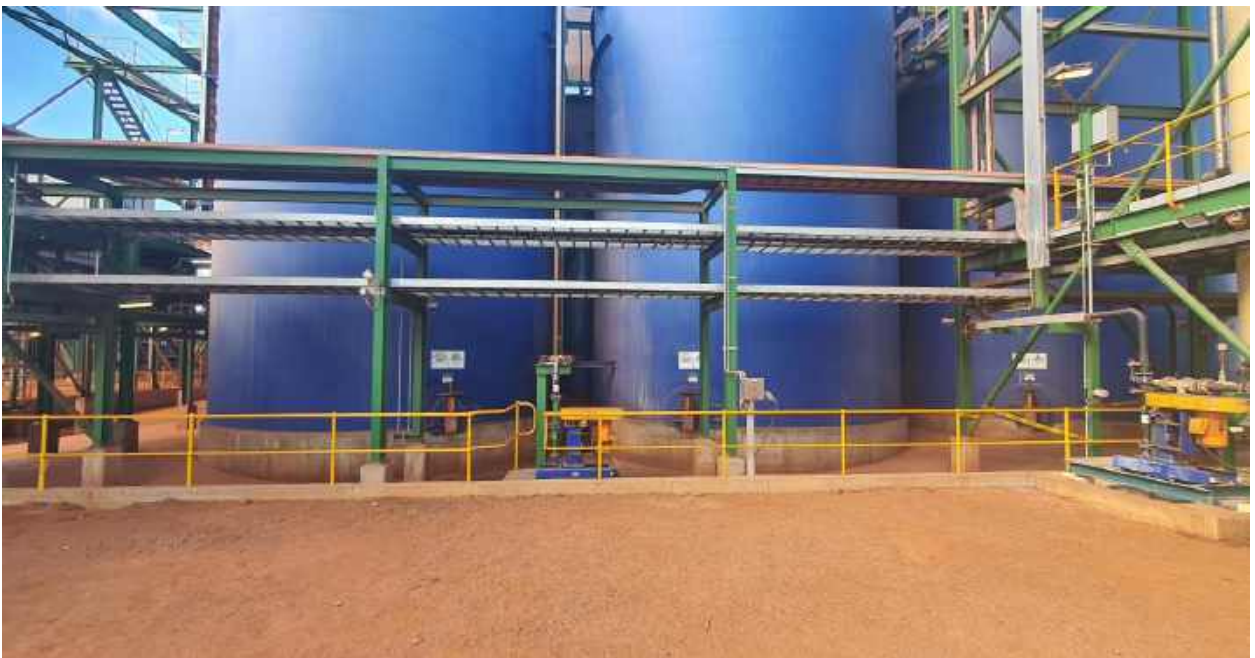
Photo 9 CIP circuit bund – CIP vats
