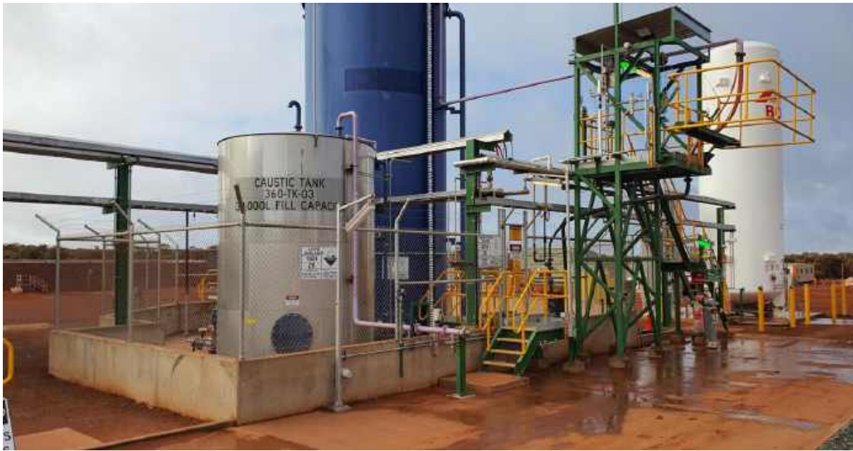
Photo 3 Caustic alkali tank bunding
