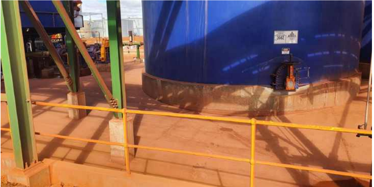
Photo 8 CIP circuit bund – CIP vats
