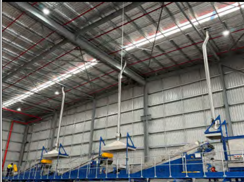
METAL TURNINGS SHREDDER AND WASH PLANT – VENT STACKS
