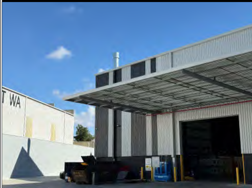
EXTERNAL VIEW - PLASMA-CUTTING STATION EXTRACTION VENT STACK
