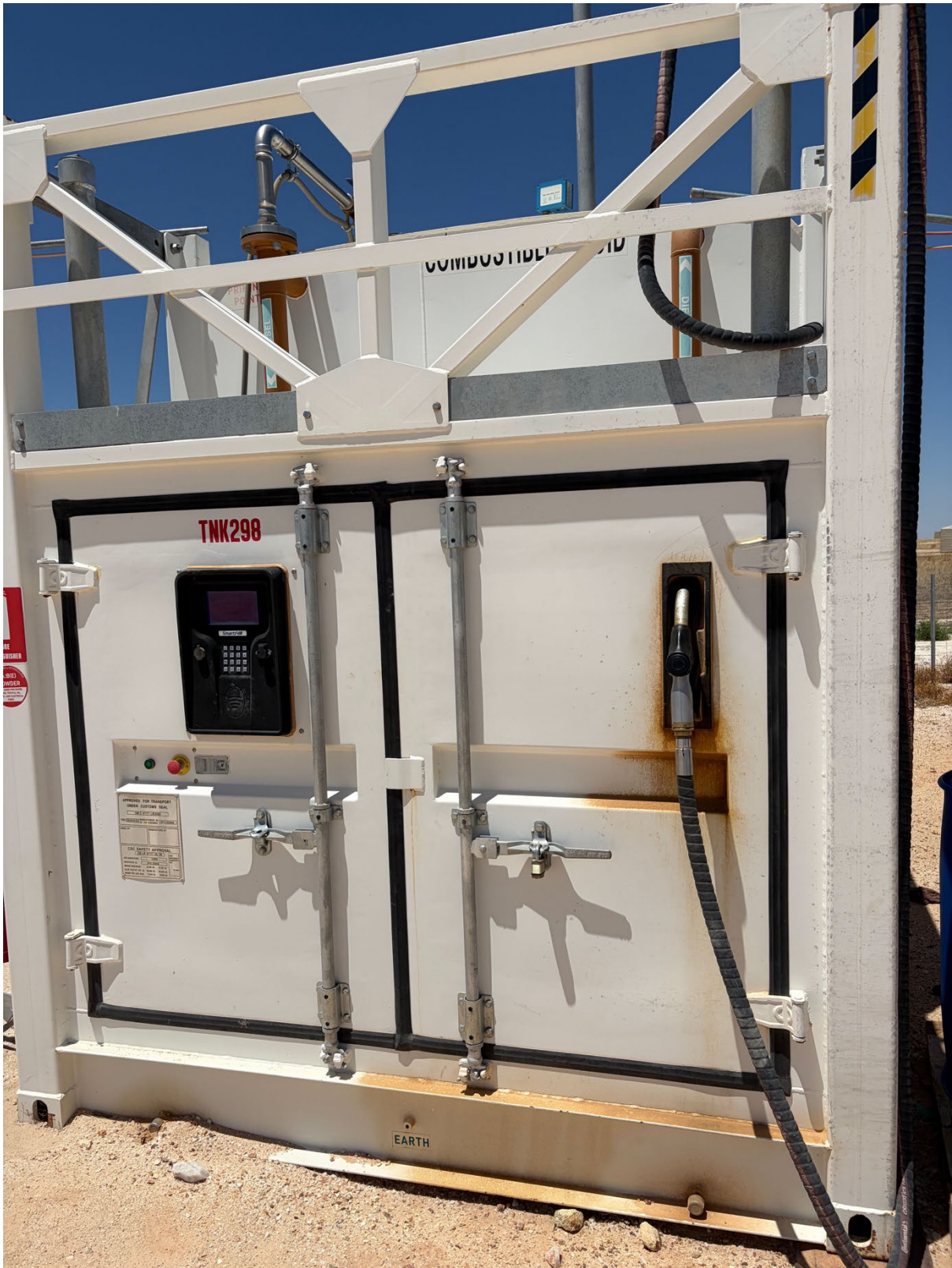
20,000 litre fuel storage- double skinned with electronic security and despatch metering.
