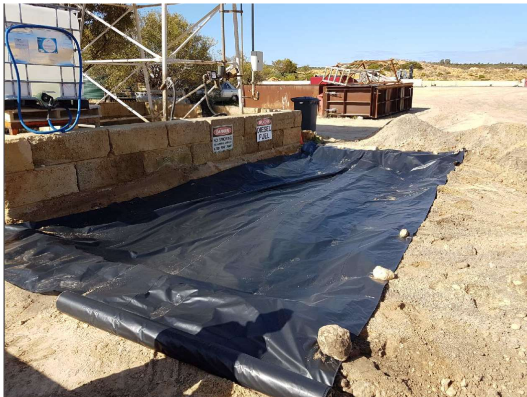
Figure 1: Diesel storage tank facility.
