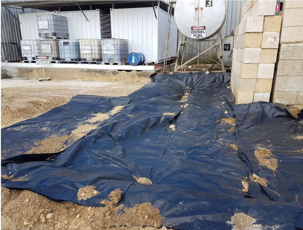
Figure 2: Diesel storage facility for generators.
