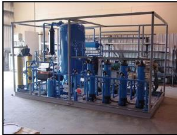
Figure 1: Photo of skid mounted DFO plant
