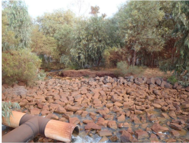
Figure 12: Example of a ‘T-piece and rip-rap’ type discharge outlet at Yandicoogina DO8 (RTIO, March 2017a)
