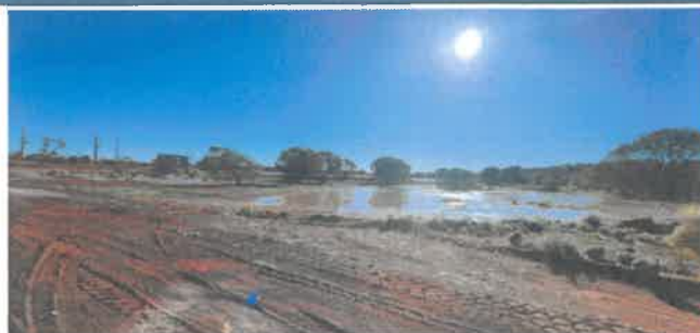
Figure 5. TSF3 pipeline spill showing car across the spill at night containment and scour pit in the background
