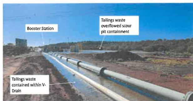
Figure 3: Photo of TSF3 Pipeline Staff looking west along pipeline 2022 scour pit
